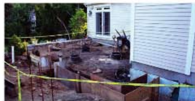
SHOWN HERE: Poor construction led to drainage problems which caused this patio to collapse. The landscape architect corrected the problem by excavating below the basement floor level. Crushed footing drains and septic piping were replaced and a drainage mat was installed against the foundation. New backfill material was distributed and compacted in lifts to allow concrete caissons to rest on undisturbed grade providing a solid support for the concrete patio slabs.
